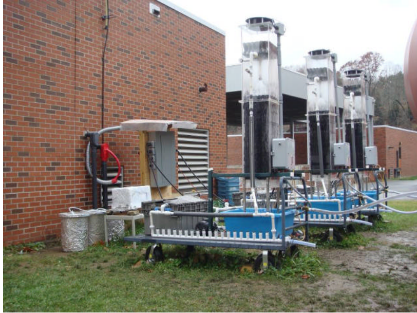
Figure 1. The pilot-scale cooling towers employed at Franklin Township Municipal Sanitary Authority (Murrysville, PA) to study corrosion, scaling, and biofouling when secondary effluent is used as the cooling tower makeup water.
