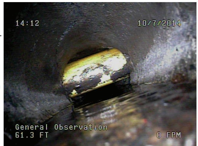
Gas Line Bored Through a Sewer Lateral
